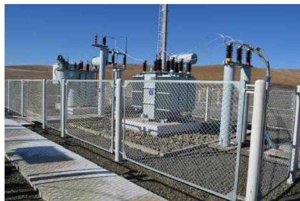
Figure 2.16 35kV electric arc dissipating coil
