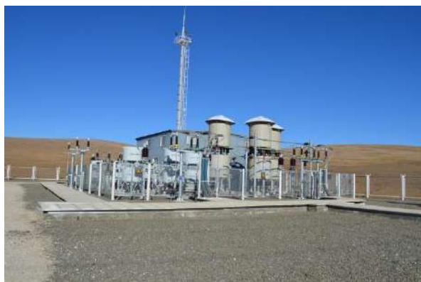
Source: Assessment team of supplementary clarification of DEIA, 2016 Figure 2.15 35kV voltage stabilizer
