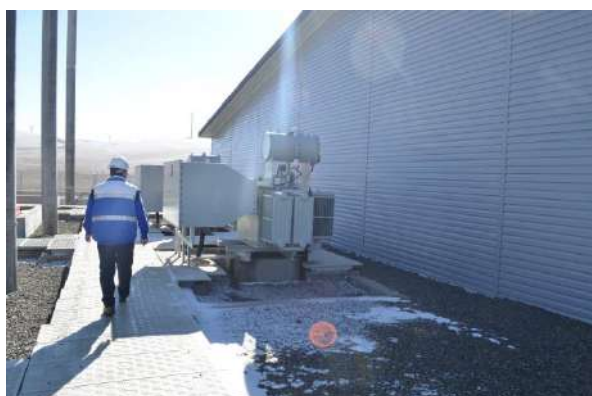
Source: Assessment team of supplementary clarification of DEIA, 2016 Figure 2.17 35/0.4kV domestic usage transformer
