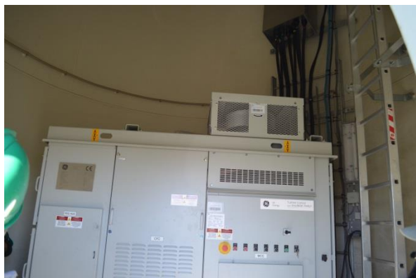
Source: Assessment team of supplementary Figure 2.9 Inverter inside the tower
