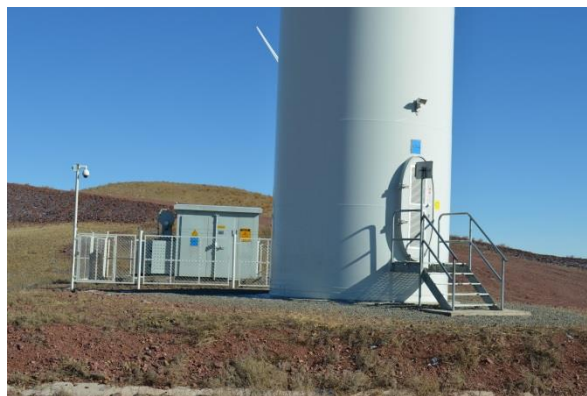
clarification of DEIA, 2016 Figure 2.10 35/0.69 kV amplifying transformer outside the tower
