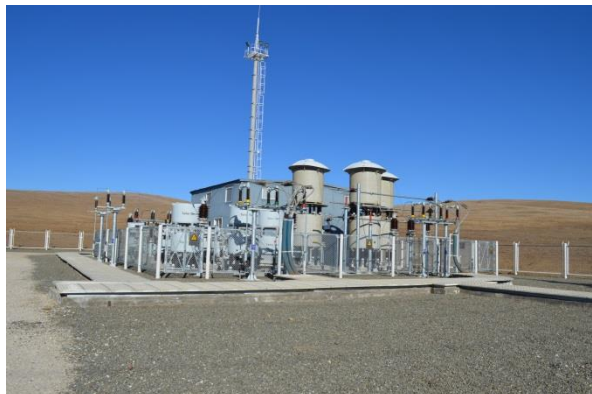
Source: Assessment team of supplementary clarification of DEIA, 2016 Figure 2.15 35kV voltage stabilizer
