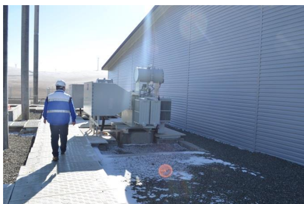
Source: Assessment team of supplementary clarification of DEIA, 2016 Figure 2.17 35/0.4kV domestic usage transformer
